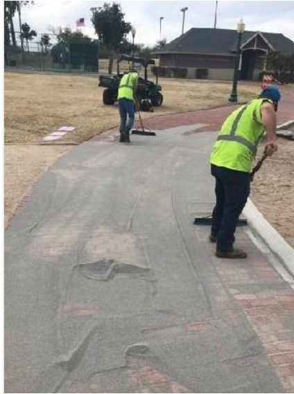
Above, crews install sand to prepare for refurbishing the pavers at South Lake.
