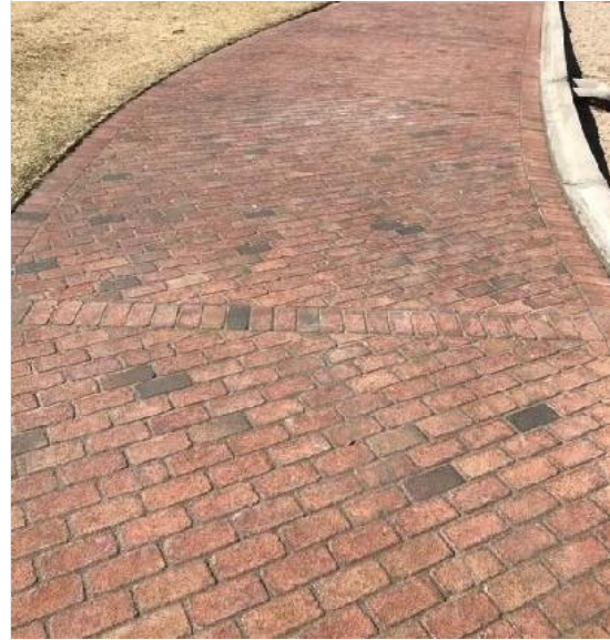
Above is a section of pavers where sand has been installed and the area completed.
